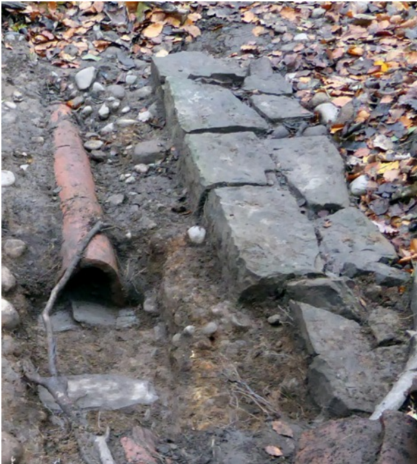
Eastern foundation of north wall. 50 cm wide and using larger sandstone blocks on outer side of wall.
