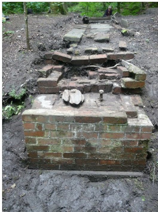
The southern bridge support looking from the Trub Brook towards the house. Two large iron bolts held a timber walk way a fragment of which is still in place.
